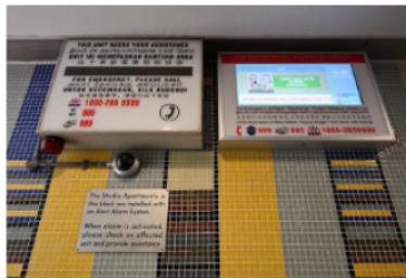
When the AAS is activated, the affected unit number will start blinking on an electronic board at the lift lobby. A siren on the first floor will also be triggered.
