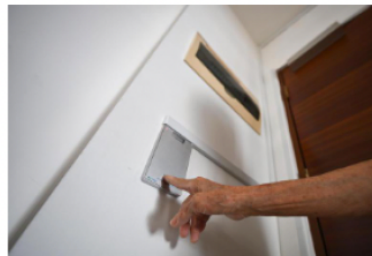
Residents have access to an electronic panel behind the main door to switch off the alarm in case of accidental activation.
